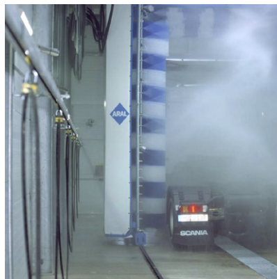
Hose-transportation in a truck washing facility
