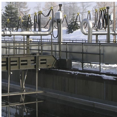
Main power supply of a longitudinal scraper bridge in a waste water treatment plant
