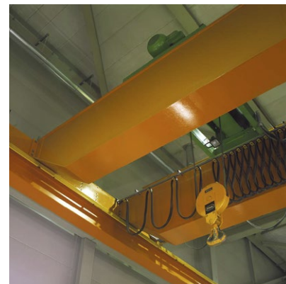
Power supply of the crab on an overhead bridge crane
